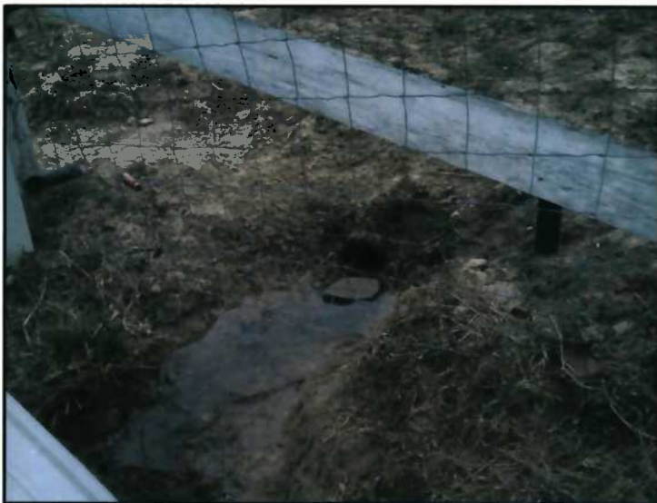
19) 4" CPP (Culvert Exit) for WL 2 overflow
