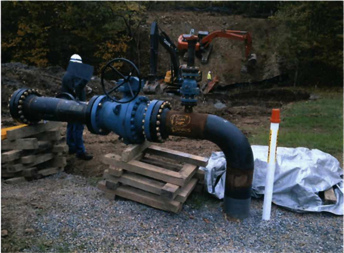
Typical above ground riser valve
