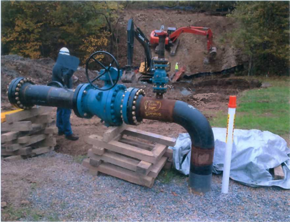
Typical above ground riser valve
