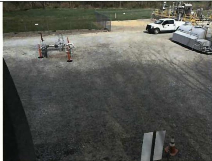
Photo: 3 Date: 4-28-2015 Comments: Overview of location of new compressor building, approximately 40 feet in front of the existing building, facing ENE.
