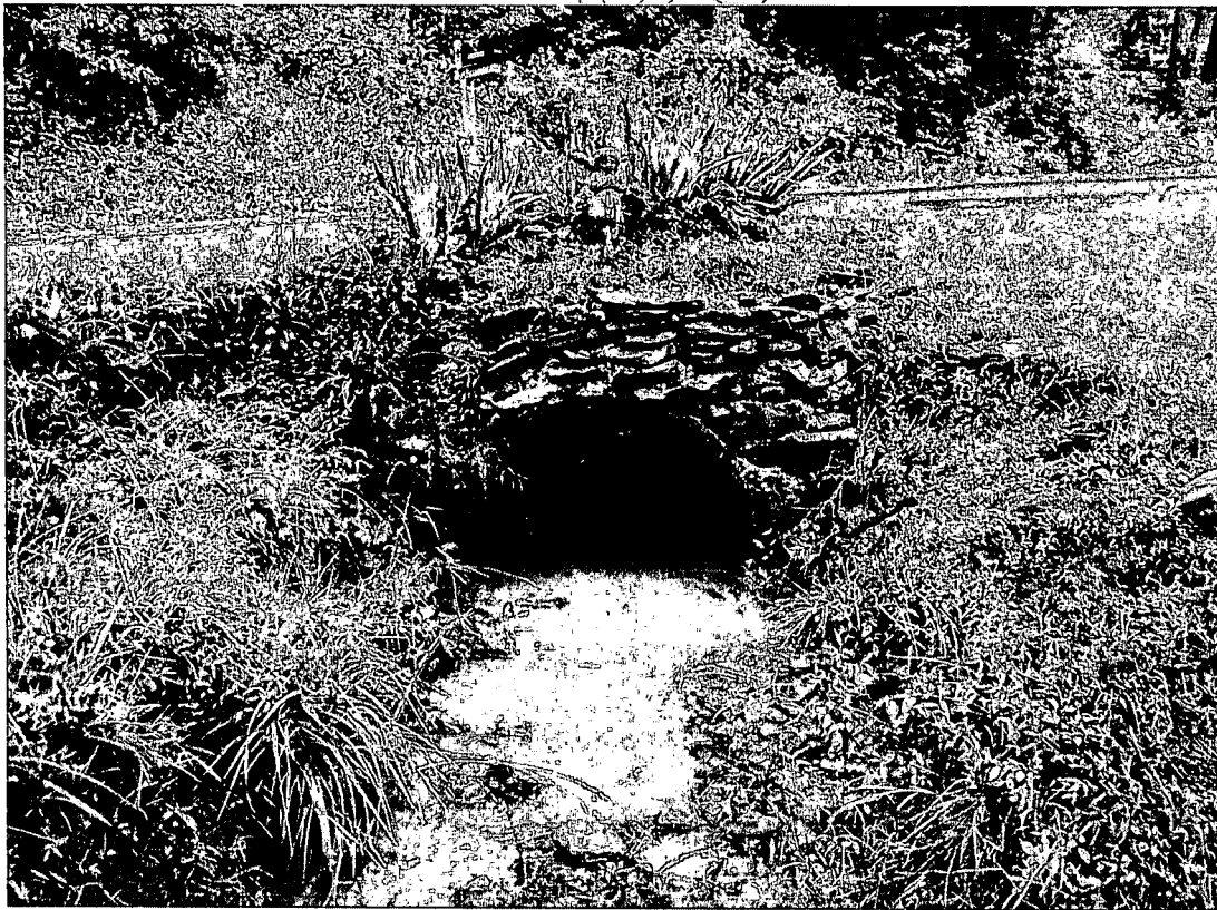
Photo 2. Facing North looking at the outlet for the existing, channelized, ditched stream to be upgraded. County Route 4 can be seen in this photo.
