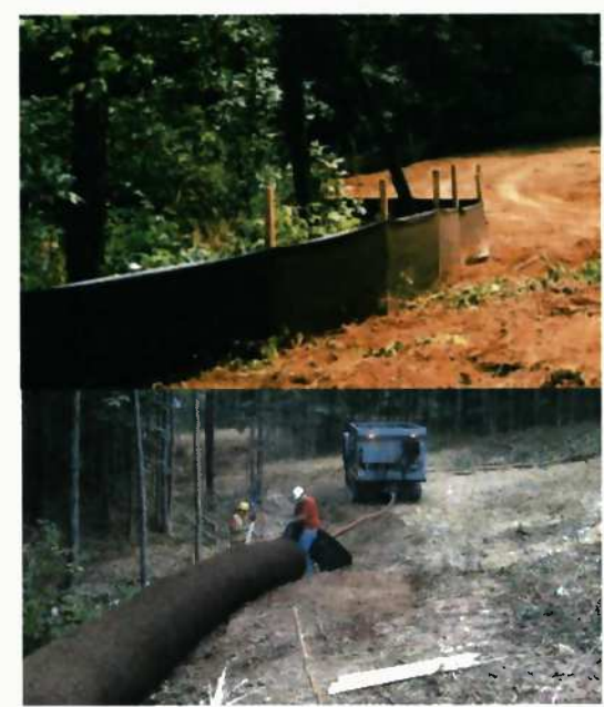
37B SUPPLEMENTAL 404 CWA BMP CONTROLS NTS DETAIL PROVIDED BY ANTERO MIDSTREAM LLC
