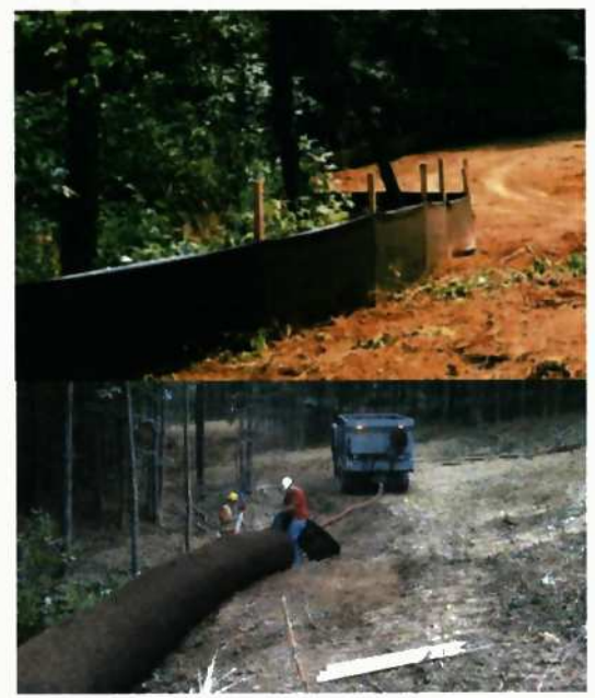
PHASE II: THIS CONTROL CONSISTS OF TYPICAL SILT FENCE, SUPER SILT FENCE, OR FILTER SOXX. THIS CONTROL WILL BE INSTALLED AS DESCRIBED IN THE PREVIOUS SECTIONS. THIS CONTROL WILL TYPICALLY BE USED WHEN WETLANDS OR STREAMS ARE LOCATED WITHIN 100 FEET OF THE DISTURBED AREA.
