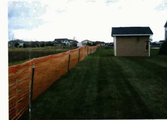
PHASE I: THIS IS ESSENTIALLY ORANGE SAFETY FENCE LIKE SHOWN ABOVE. THIS MEASURE IS PUT IN PLACE TO LET CONTRACTORS KNOW THAT NO WORK IS TAKE PLACE BEYOND THIS POINT. THIS CONTROL IS TYPICALLY UTILIZED WHEN THERE IS A WETLAND OR STREAM LOCATED IN THE AREA BUT NOT WITHIN APPROXIMATELY 100 FEET OF THE DISTURBANCE.
