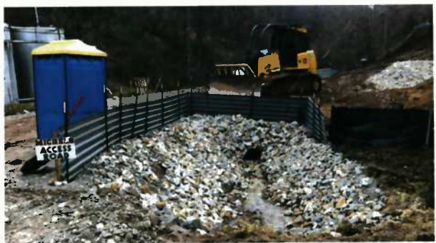
PHASE III: THIS CONTROL CONSISTS OF METAL Q-DECKING WHICH IS STOOD ON ITS EDGE AND SECURED TO METAL POSTS. THIS CONTROL IS USED TO PREVENT SOILS OR GRAVELS FROM ENTERING STREAMS OR WETLANDS DURING CONSTRUCTION. THE DECKING CAN BE BURIED OR USED IN CONJUNCTION WITH OTHER E&S METHODS. THIS CONTROL IS USED IN AREAS WHERE STREAMS OR WETLANDS ARE WITHIN APPROXIMATELY 50 FEET OF THE DISTURBED AREA. IF THE METAL DECKING IS BURIED NO OTHER E&S CONTROLS ARE REQUIRED, BUT IF THE DECKING IS PLACED ON TOP OF THE GROUND SURFACE AND ADDITIONAL E&S CONTROL SUCH AS SILT FENCE OR SILT SOXX WILL BE USED TO PROTECT THE GAPS BETWEEN THE BOTTOM OF THE DECKING AND THE UNEVEN GROUND SURFACE.
