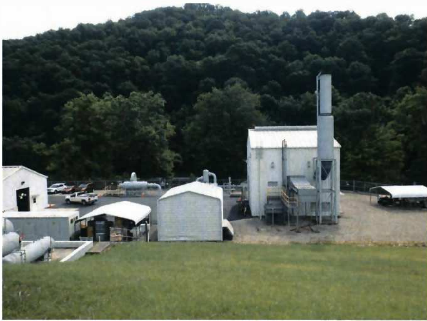
PHOTO 1 Existing compressor station.
