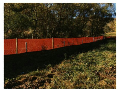
43C SUPPLEMENTAL 404 CWA BMP CONTROLS NTS DETAIL PROVIDED BY ANTERO MEDITERRAN LLC
