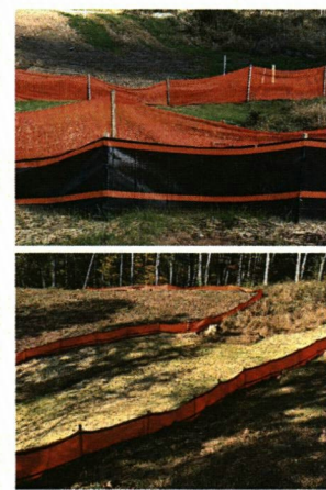
43B SUPPLEMENTAL 404 CWA BMP CONTROLS NTS DETAIL PROVIDED BY ANTERO MEDITERRAN LLC
