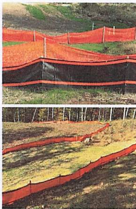
PHASE II: THIS CONTROL CONSISTS OF TYPICAL SILT FENCE, SUPER SILT FENCE, OR FILTER SOCK. THIS CONTROL WILL BE INSTALLED AS DESCRIBED IN THE PREVIOUS SECTIONS. THIS CONTROL WILL TYPICALLY BE USED WHEN WETLANDS OR STREAMS ARE LOCATED WITHIN 100 FEET OF THE DISTURBED AREA.
