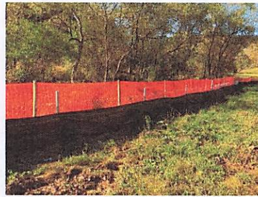
PHASE III: THIS CONTROL CONSISTS OF SUPER SILT FENCE WITH ORANGE CONSTRUCTION FENCE ACTING AS THE VISIBLE PORTION OF THE BARRIER. THIS CONTROL IS USED TO PREVENT SOILS OR GRAVELS FROM ENTERING STREAMS OR WETLANDS DURING CONSTRUCTION. THE SUPER SILT FENCE CAN BE USED IN CONJUNCTION WITH OTHER EAS METHODS. THIS CONTROL IS USED IN AREAS WHERE STREAMS OR WETLANDS ARE WITHIN APPROXIMATELY 50 FEET OF THE DISTURBED AREA.
